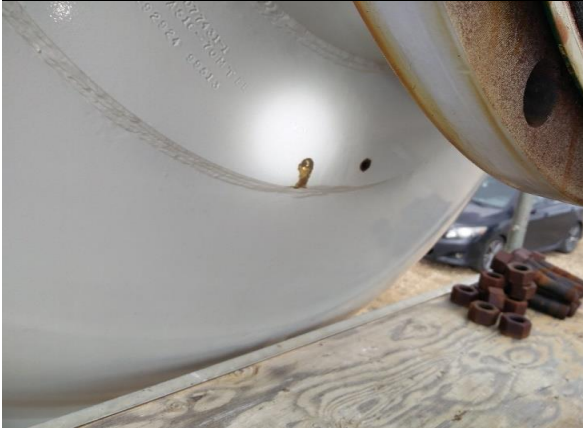
Photo 13 Description: Split repad on manway weep hole still grease
