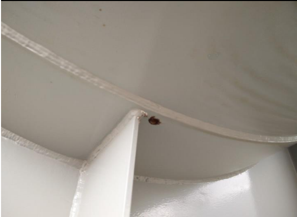
Photo 15 Description: Saddle weep hole still with grease
