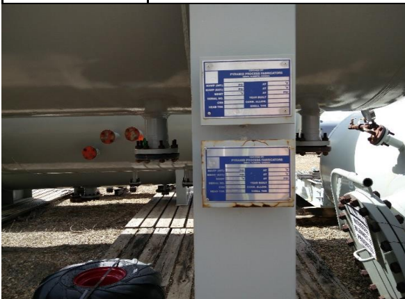
Photo 3 Description: 2 nameplates, 1 metric and 1 SAE
