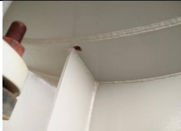
Photo 16 Description: Saddle weep hole still with grease
