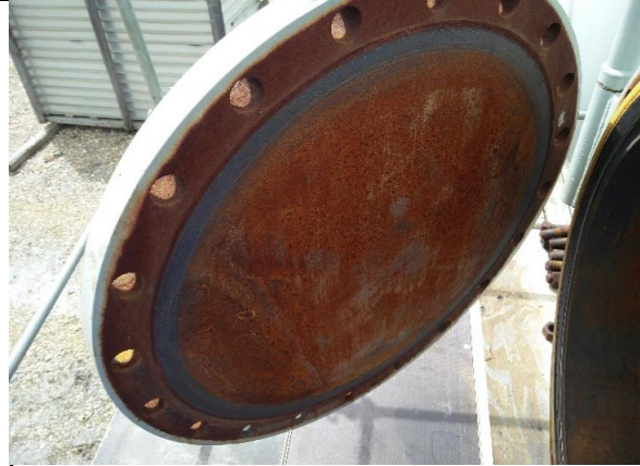
Photo 8 Description: Manway blind slight surface rust
